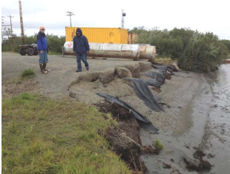
Figure 5-5 Photo of Eroding Rip-Rap Along the Qinaq River (ADEC 2012)
