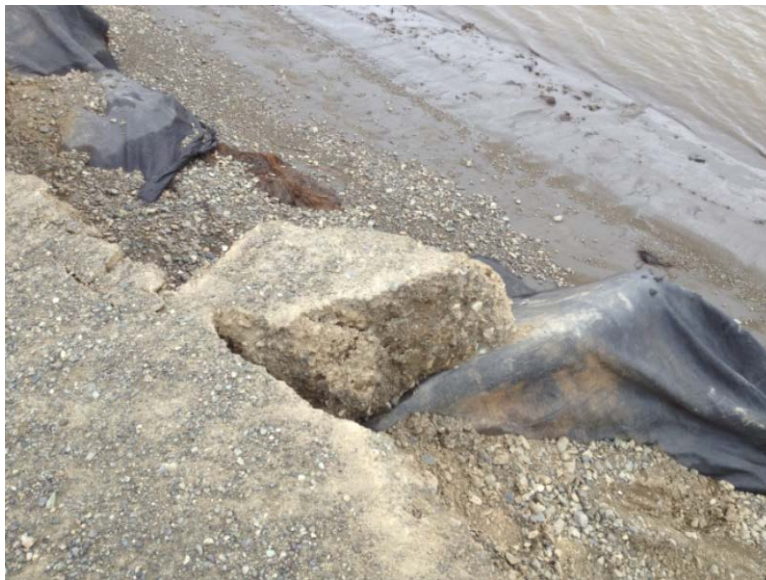
Figure 5-6 Close-Up photo of Eroding Rip-Rap Along the Qinaq River (ADEC 2012)
